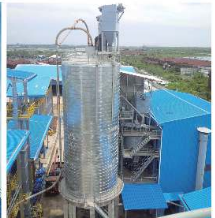
9. Silo auxiliary installation
