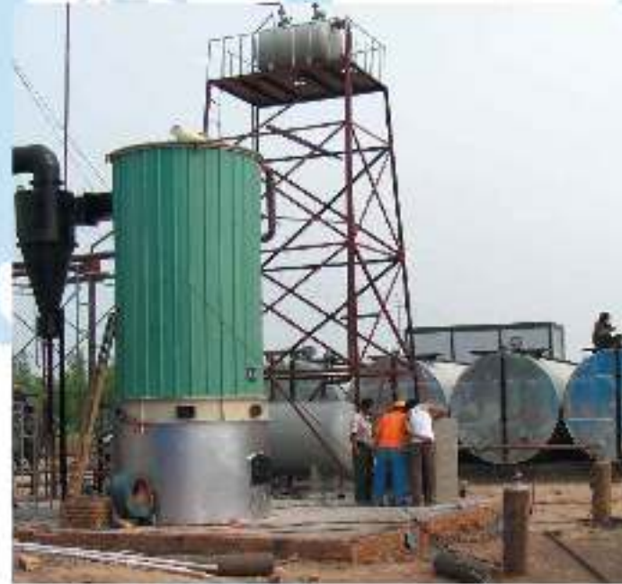
Coal Fired Thermal Oil Boiler In Kazakhstan Asphalt Heating Plant
