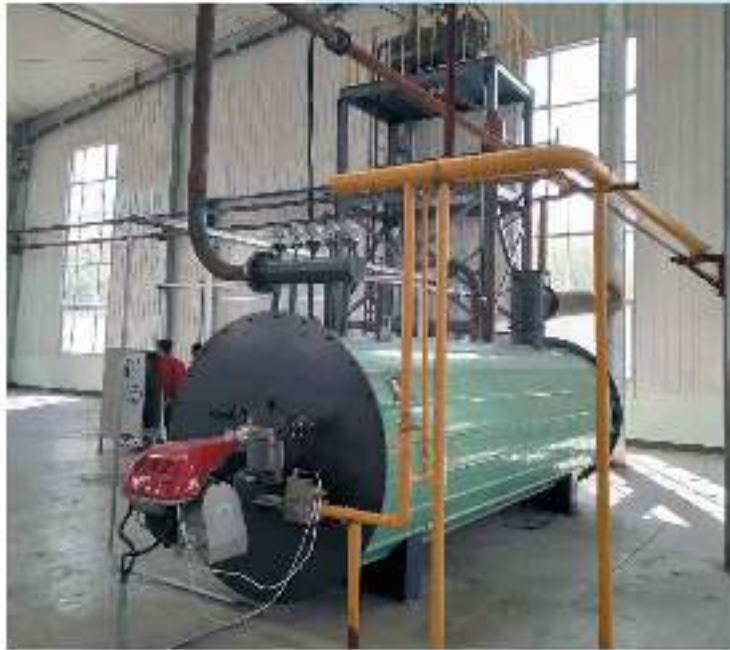
Thermal Fluid Heater In Argentina Chemical Plant
