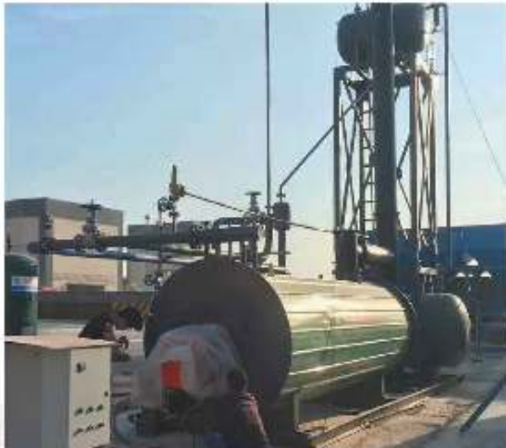
Thermal Oil Heater in UAE Lubricant Factory
