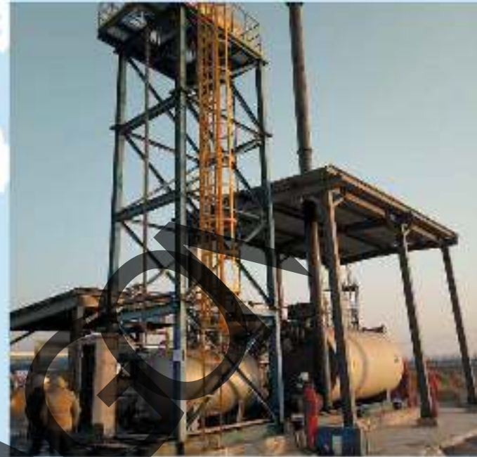
Gas Fired Thermal Oil Boiler In USA G.E. Company(China Branch Company)
